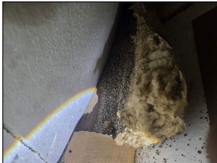
90. Possible asbestos containing materials
