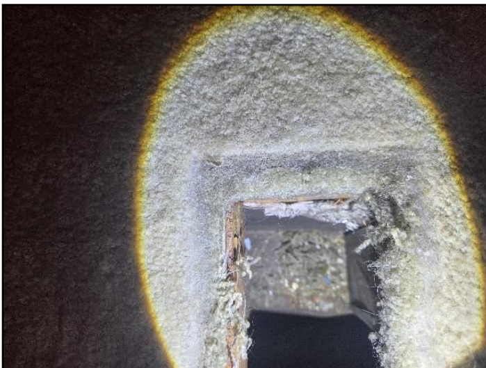
80. Possible asbestos containing materials
