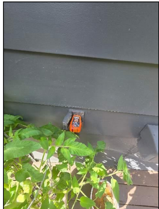
39. GFCI/GFI needed (Ground Fault Circuit In
