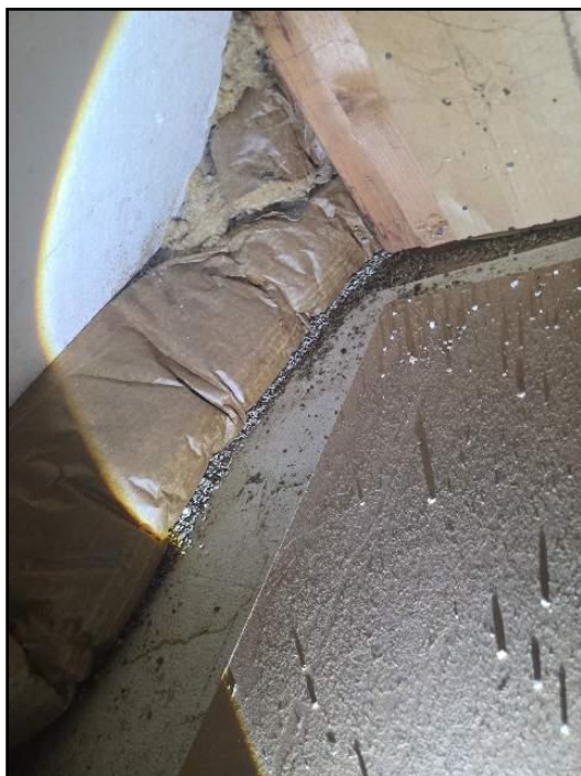
91. Possible asbestos containing materials
