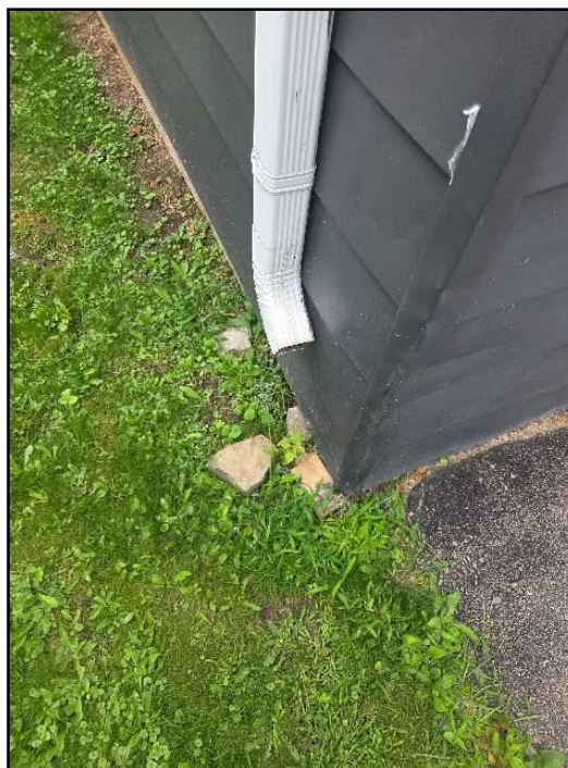
10. Discharge too close to building
