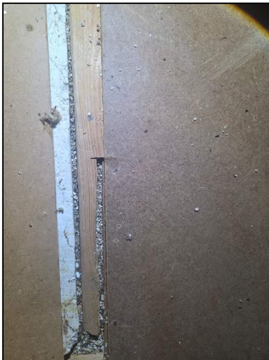
87. Possible asbestos containing materials
