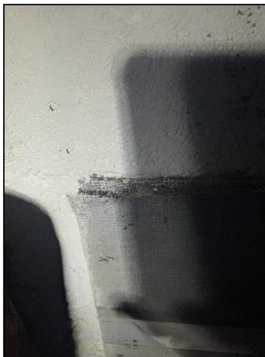
83. Possible asbestos containing materials
