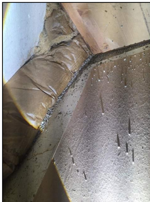
92. Possible asbestos containing materials
