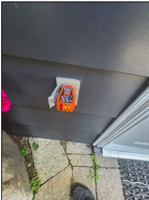
38. GFCI/GFI needed (Ground Fault Circuit In
