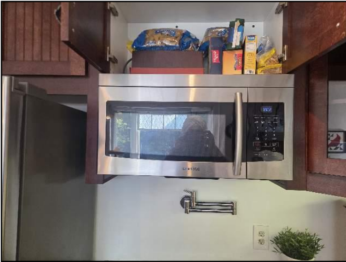
75. Not vented to exterior
