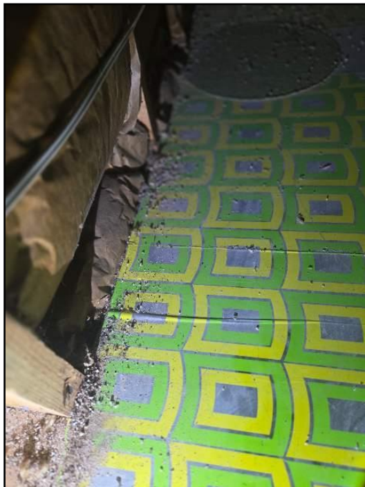
89. Possible asbestos containing materials
