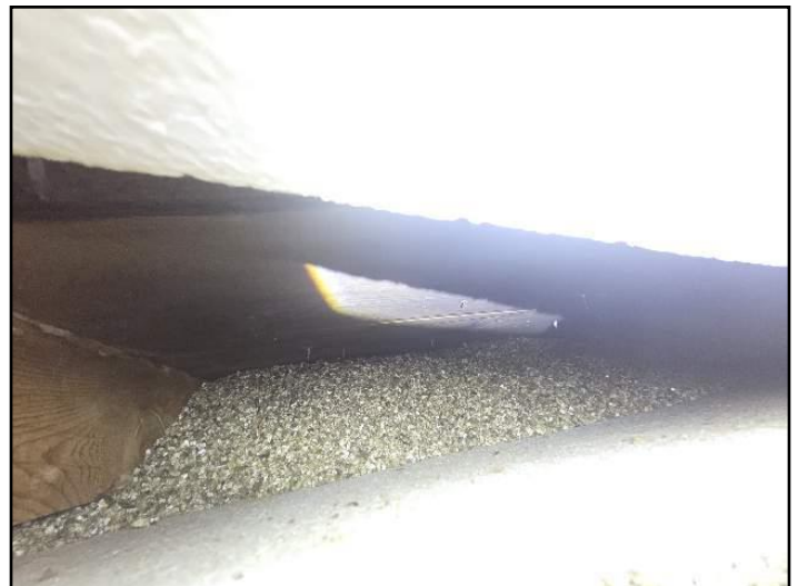
88. Possible asbestos containing materials
