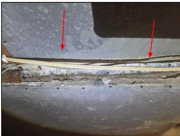
82. Possible asbestos containing materials
