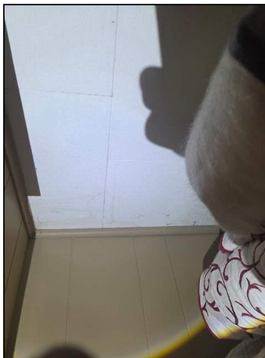
84. Possible asbestos containing materials
