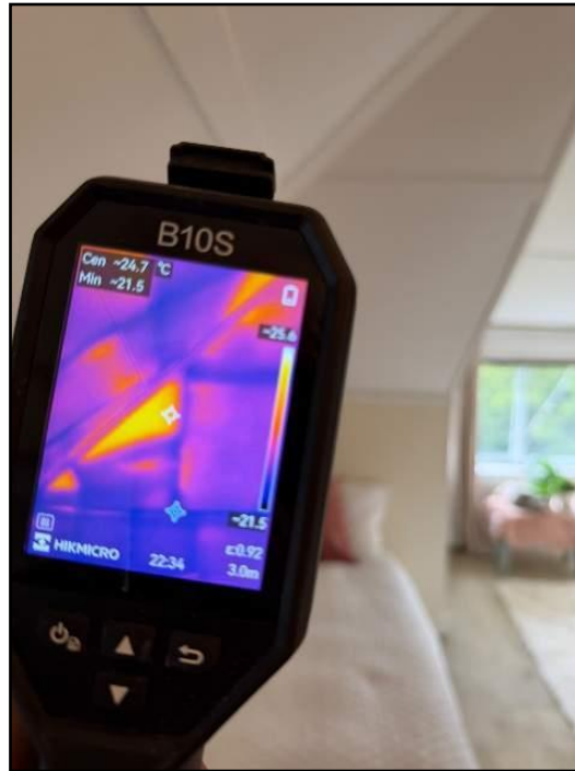
52. Gaps or voids
