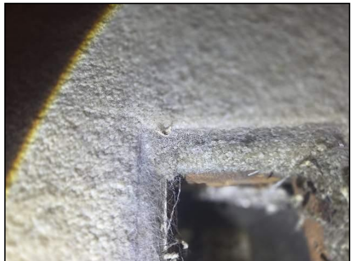
81. Possible asbestos containing materials
