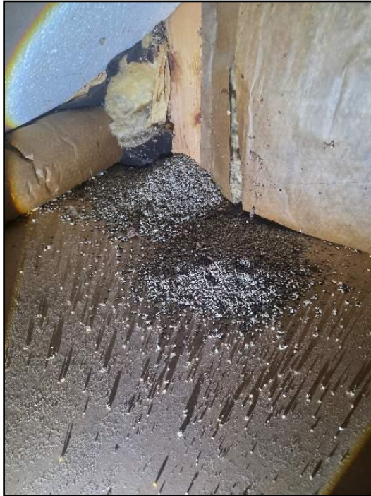
85. Possible asbestos containing materials
